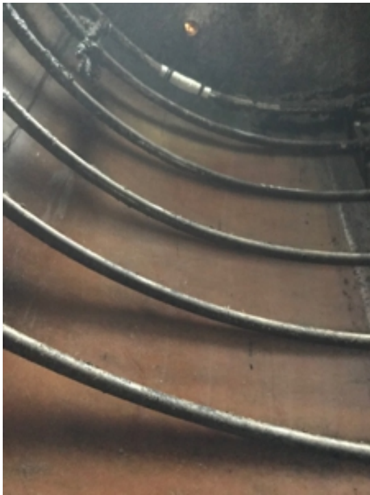
Damaged pipe located at the top of the heating tank, as seen once wrapped in SylWrap HD
