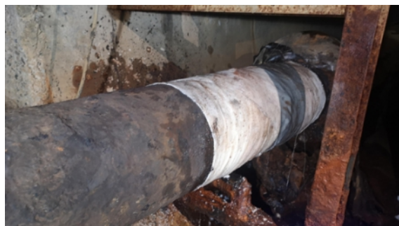
Section two of the pipe repaired and protected with an overwrapping of SylWrap HD
