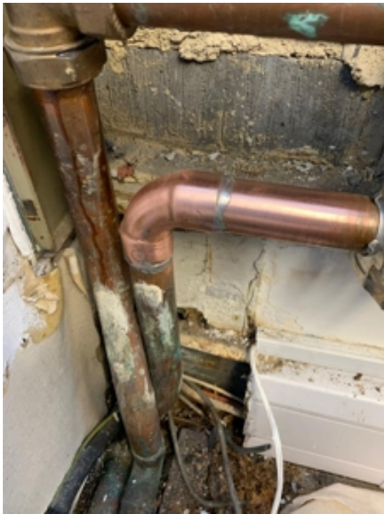
The copper pipe having been polished but prior to the application of Wrap & Seal
