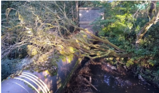
One of the 20m pipe bridges requiring repair
