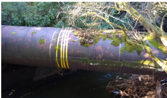
Yellow tape shows a previously failed repair attempt
