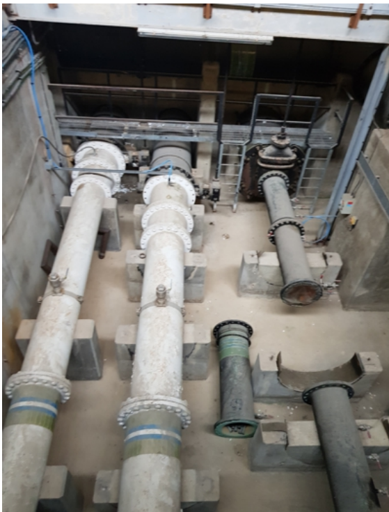
Pipework in the valve chamber
