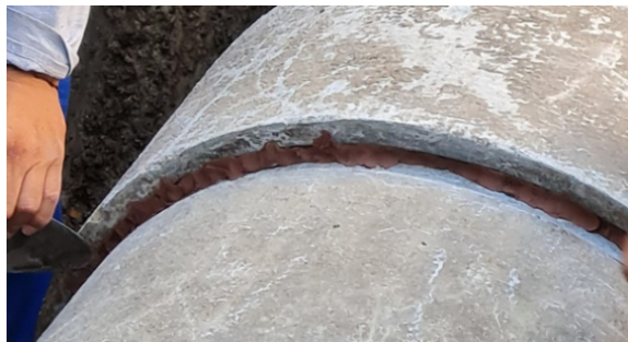
Superfast Copper sealed the gaps between the sleeve and the surface of the pipe
