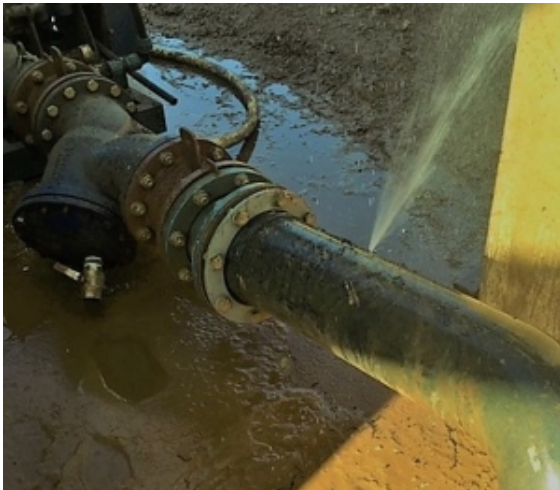
Jet of pressurised water escaping from the pinhole leak caused by a pierce to the plastic pipe
