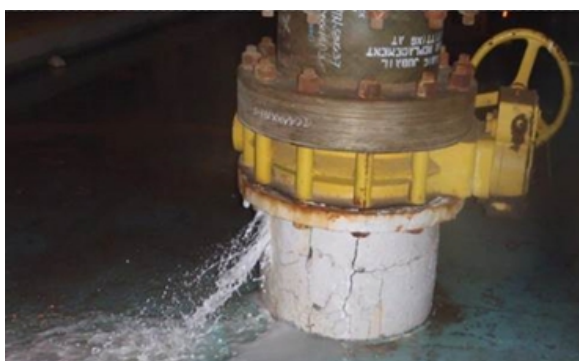
Water escaping from numerous cracks in the stub at 4 bar pressure, causing flooding
