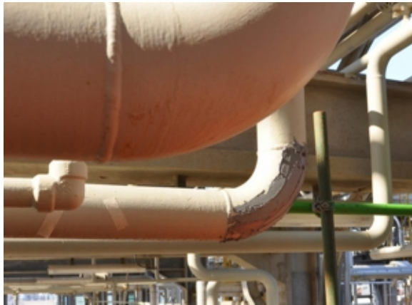
The weakened elbow joint was coated with Industrial Metal Epoxy paste for reinforcement
