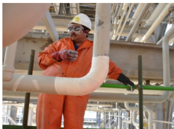
SylWrap HD was used to complete the repair, setting rock hard for an impact resistant layer of protection
