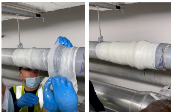
SylWrap HD provided a rock hard, protective sleeve to complete the repair
