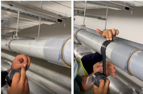
The pipe was leaking from the left hand side of the joint with the application of Wrap & Seal starting 100mm away to build up a ridge towards the step
