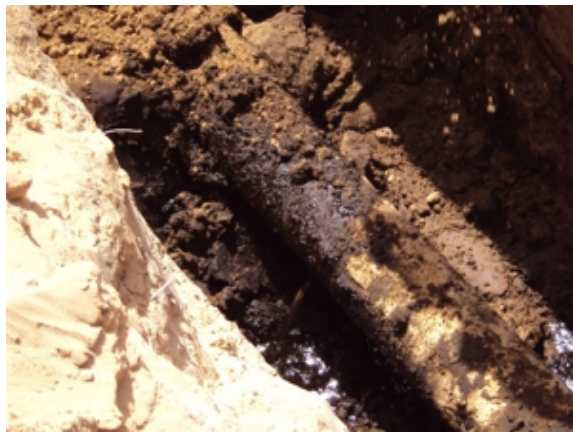
Pipe covered in dirt, rust and oil following excavation
