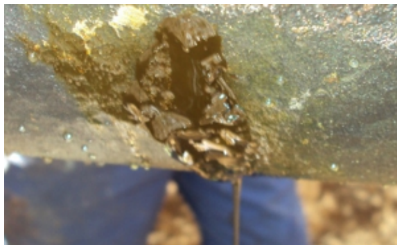
Oil was escaping from a crack caused by corrosion
