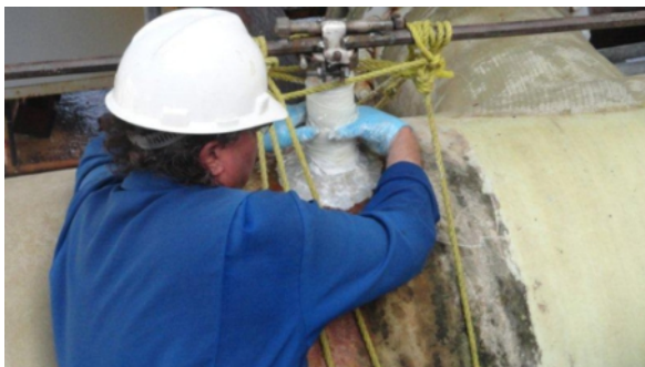
Further reinforcement was given to the plug and AB Original by seven layers of SylWrap HD
