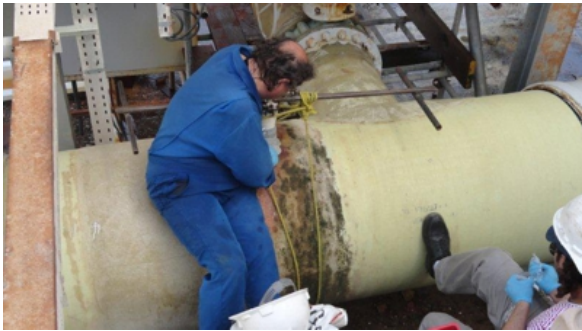
The pipe surface had been damaged and weakened by the 5 metre high water discharge through the hole
