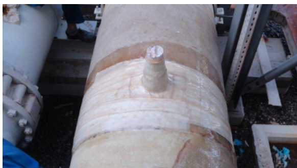
Repair was completed by encompassing weakened section of pipe with a protective sleeve of SylWrap HD, strengthening it against future breaches
