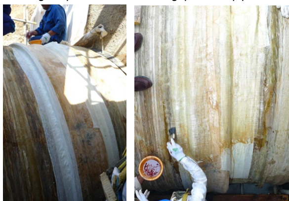
Fibreglass Tape saturated with E190 Brushable Epoxy layered over the ring to build a composite patch repair
