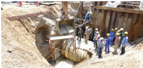
The chamber housing the leaking section of partly buried line was drained after it was flooded by water escaping when the system was first turned on
