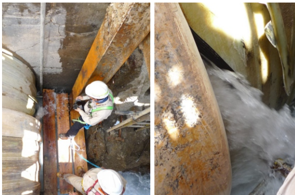
Minimal flow was restored to identify the leak cause, found to be gaps at each end of a connecting ring
