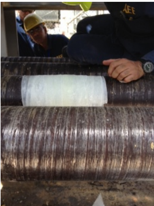
The completed repair enabled the Power Station to operate at full capacity after Hurricane Maria hit Puerto Rico
