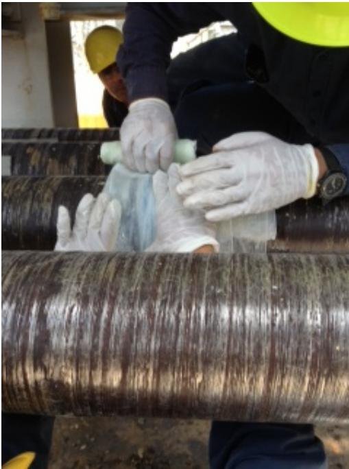
SylWrap HD is applied after the crack had been sealed using Wrap & Seal
