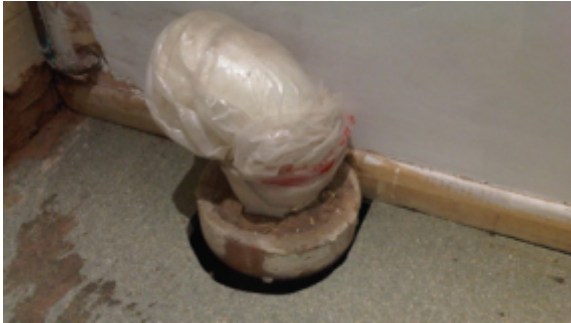
Gapping between the pipe and the floor needed filling with the crack 50mm wide at its biggest point
