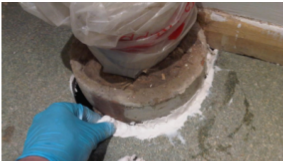
Sylmasta AB Original was kneaded by hand and then pushed into the crack, filling the gap
