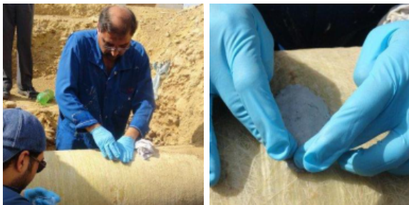
Superfast Steel was pushed onto the pipe to fill the imperfections in the line
