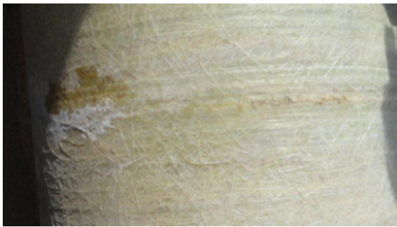
The external surface of the GRP pipe suffering from heavy scoring with the potential to lead to breaches
