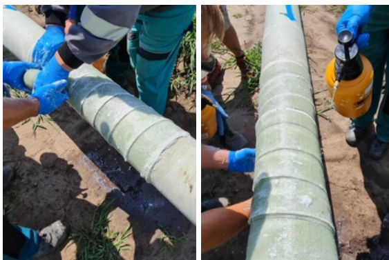
After being smoothed, SylShield cured to form an ultra hard shell protecting the steel pipe
