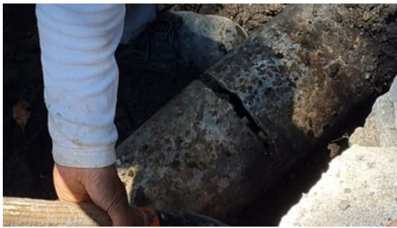
A 15mm crack was discovered in the cement coating of the pipe, although no leakage was detected
