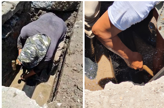
As the cement coating was removed, water began spraying from a 80mm long split in the steel pipe
