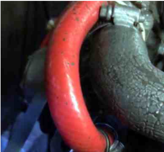
The pinhole was on a section of red coloured rubber pipe where access was severely restricted
