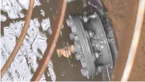
The pipe stub was difficult to access at the bottom of a chamber surrounded by metalwork
