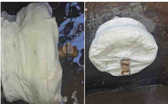
SylWrap Bandage was wrapped around the stub and smothered over the flange plate for protection
