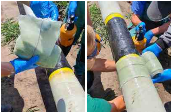
SylShield was activated with water and then wrapped over heat shrink sleeves covering the welded joints
