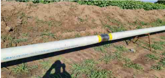
Sections of pipe were welded together (black area) to fabricate the line above ground prior to HDD
