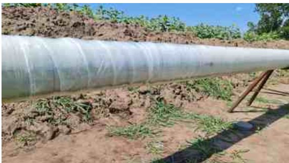
Once the line had been protected, it was ready to be pulled through the ground and installed via HDD
