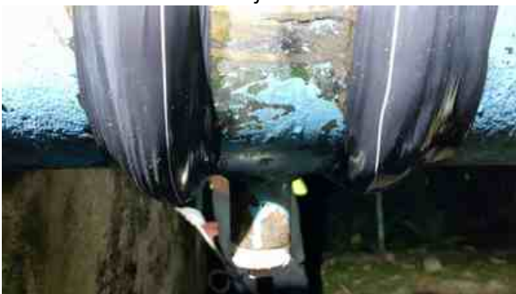
Once the joint ends had been encapsulated, Wrap & Seal was applied directly over the leak to create a ridge increasing the pressure resistance of the repair
