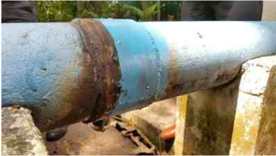
Water was seeping from both ends of the saddle joint, one of which was suffering from heavy corrosion
