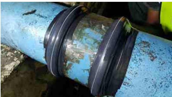
Wrap & Seal was applied to both ends of the saddle joint, successfully sealing the pipe
