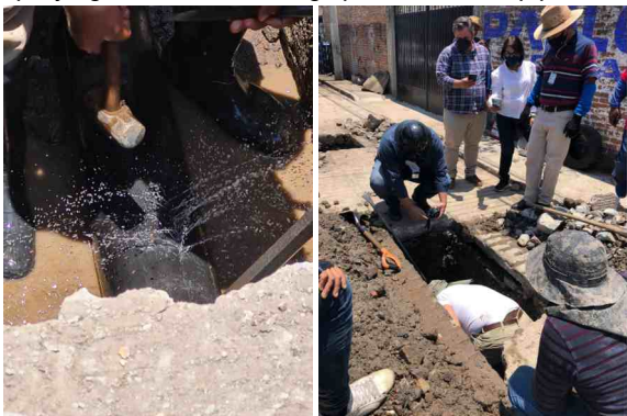
Once the coating had been fully removed, the steel pipe was sealed using a SylWrap Contractor Case
