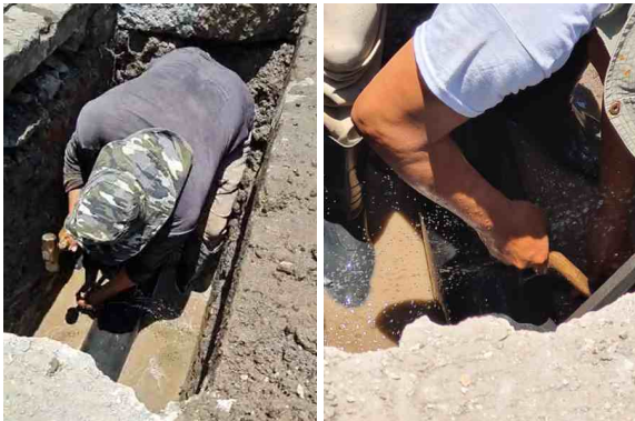
As the cement coating was removed, water began spraying from a 80mm long split in the steel pipe
