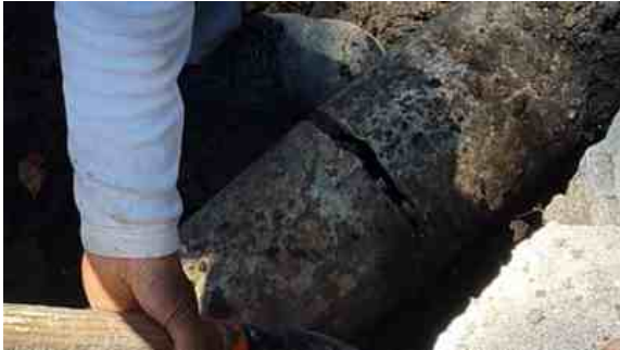
A 15mm crack was discovered in the cement coating of the pipe, although no leakage was detected
