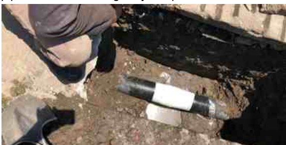
After the leak was sealed with Wrap & Seal, SylWrap Bandage replaced the protective concrete coating
