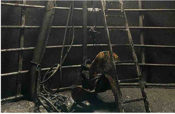
Propeller mixer blade was attached to a metal pillar inside the biodigester tank which had moved back to collide with a steel heating pipe, causing a breach
