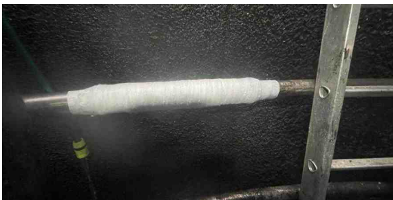
SylWrap Bandage encompassed the repair with a rockhard shield to protect against future impact from the pillar and mixer blade
