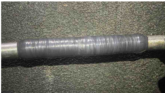
Wrap & Seal was applied along the entire 600mm length of the area which had been patch welded
