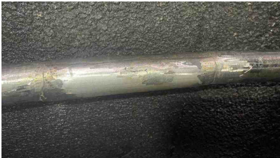
An initial repair attempt involving patch welding failed, leaving multiple pinhole leaks in the pipe
