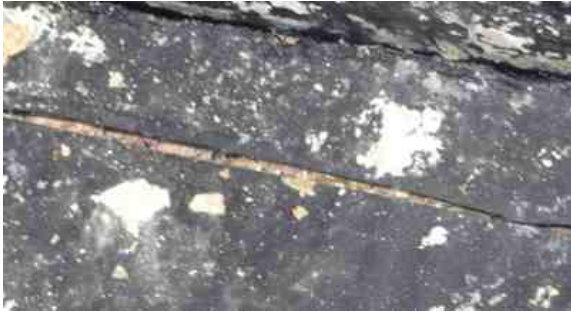
Gaps had appeared in the rubber matting, exposing the concrete lining of the tank to seawater
