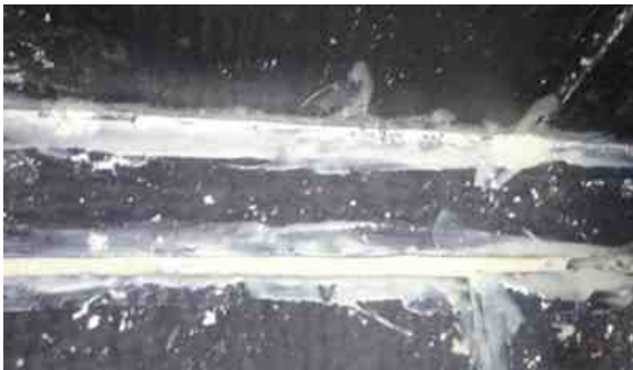
Once cured, AB formed a waterproof material sealing every gap and protecting the concrete lining beneath
