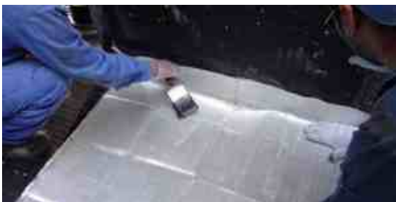
Fibreglass sheets were layered over the matting and coated with epoxy resin to create a new reinforced floor surface
