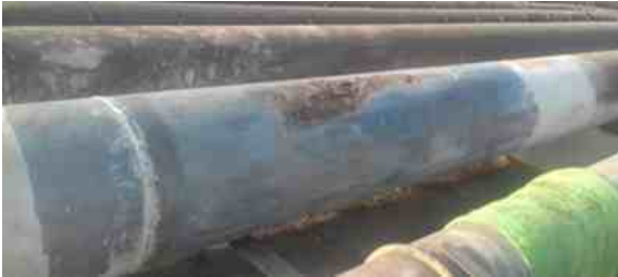
The 2 metre long section of steel pipe needed to be rebuilt where a 600mm patch of corrosion had severely weakened the line
