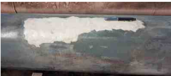
AB Original Epoxy Putty rebuilt the patch of steel pipe weakened by corrosion to its original thickness. It would offer excellent protection from further corrosion and chemical attack, and act as a sacrificial layer where necessary.
