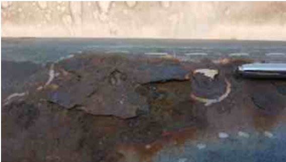
Closer inspection of the corroded area showed how much external surface damage the pipe had suffered
