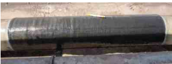
SylWrap CR was applied to a 2 metre section of the line, centred around the corroded area rebuilt using AB Original. The corrosion inhibitors in SylWrap CR provided greater protection in such an aggressive environment.
