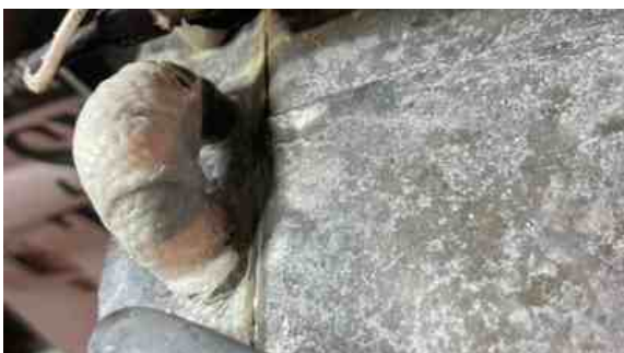
SylWrap Bandage forced the putty into the crack, creating a watertight seal and offering protection from future expansion of the pipe
