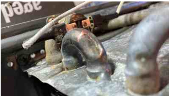
The pipe was cleaned of loose material before repair to aid adhesion with the Epoxy Putty.
