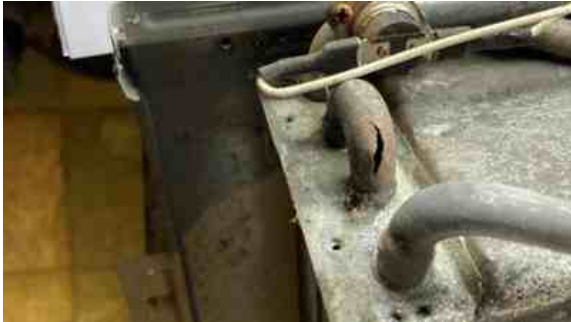
Freezing temperatures caused copper pipework in horse shower units which had not been fully drained to suffer from cracks and bursts
