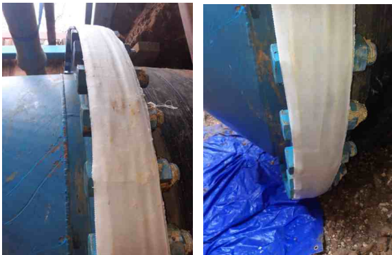
A SYL412HD Bandage was the perfect 100mm width to wrap around the flange, curing to form a rock-hard shell which tree roots would not be able to penetrate in future
