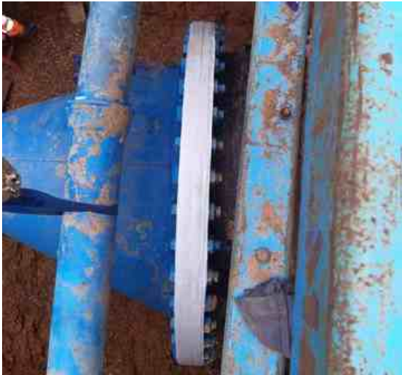
Wrap & Seal was applied all around the flange to seal the leak. It was then overwrapped with SylWrap Pipe Repair Bandage
