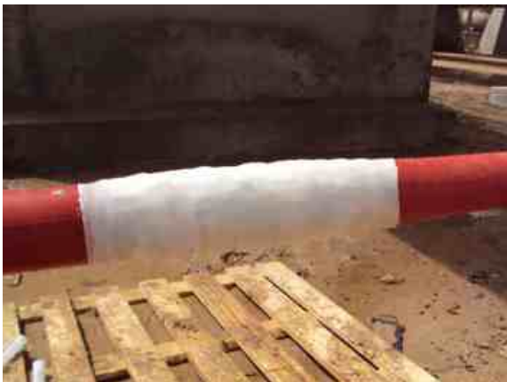
The above-ground section was successfully sealed using Wrap & Seal and then further protected with SylWrap Pipe Repair Bandage
