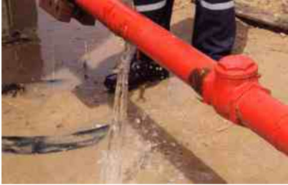
Significant levels of water were escaping the above-ground section of pipe at 5 bar pressure from a longitudinal split
