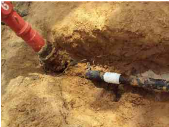
A trench was dug with enough clearance to reach the below-ground section of pipe. It was then repaired using Wrap & Seal and SylWrap Bandage
