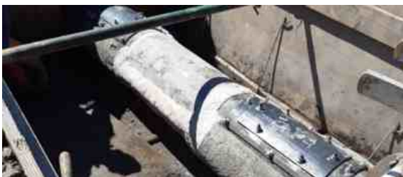
AB Original encapsulated the clamp, sealing all areas which the pipe was leaking from
