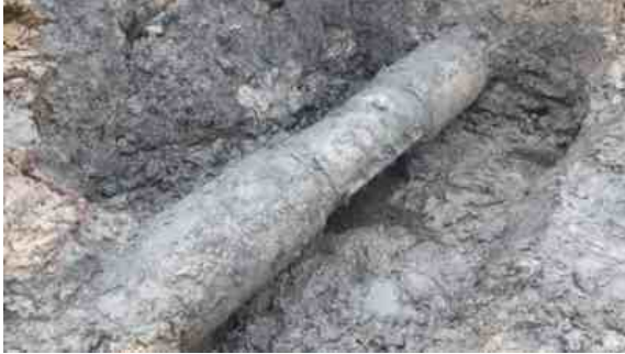
The leaking pipe ran beneath salt marshes, leaving an eight hour window with the tide out to access, excavate and clean the pipe, and seal the leak
