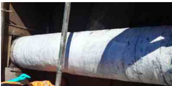
SylWrap Bandage was wrapped across the entire length of the pipe, completing the repair
