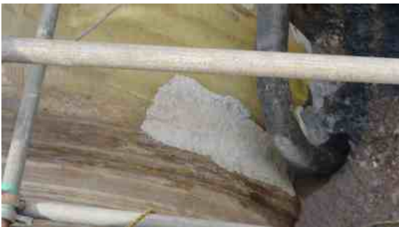
AB Original was used for larger leak areas because its longer work time allowed more putty to be mixed without the threat of premature curing
