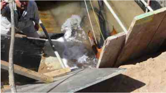
The line was isolated, excavated and re-pressurised. So much water escaped that the hole dug to access the pipe became instantly flooded
