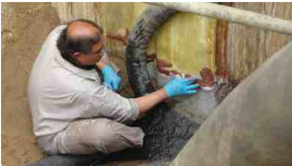
Superfast Copper sealed smaller holes in the line in five minutes
