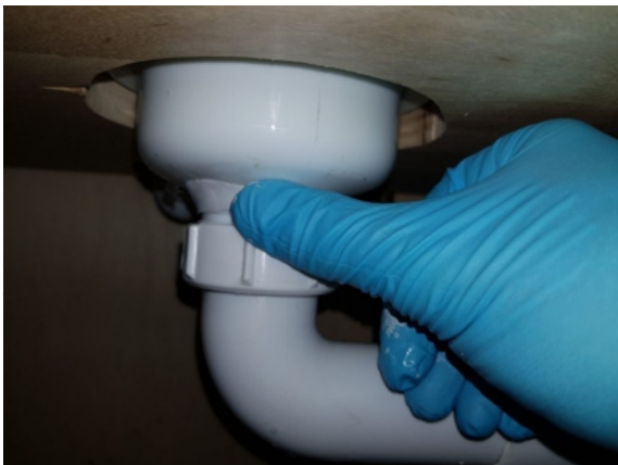
Superfast Plastic was kneaded by hand, formed into a sausage shape and pushed over the cracks in the pipe whilst the putty remained soft
