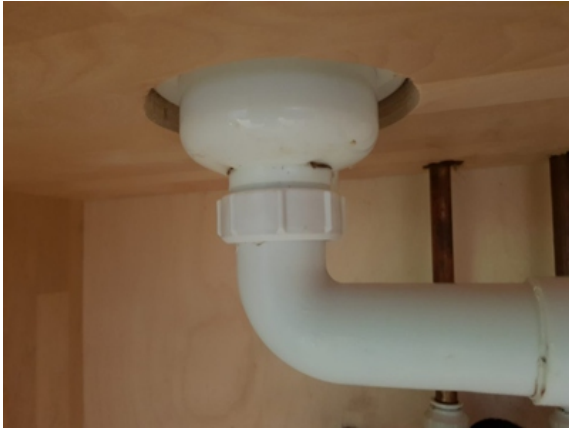
Cracks had appeared in the top of the PVC plastic drain pipe where it connected to the sink
