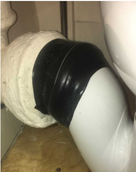
Wrap & Seal created a solid rubber ring, sealing the pipe whilst allowing it a degree of movement
