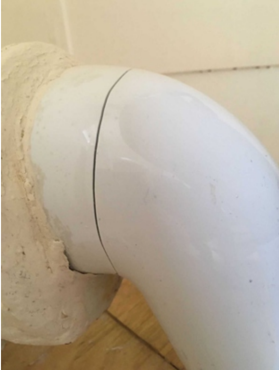
The hairline crack was around the entire diameter of the porcelain toilet soil pipe
