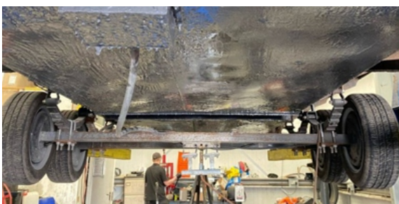
Liquid Metal was coated onto the underneath of the trailers to strengthen the brittle original metalwork and protect it from future corrosion
