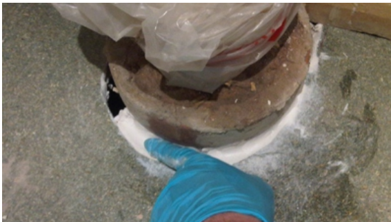
The putty was smoothed off using a little water and a filling knife as the application continued
