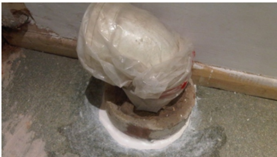
The completed repair with all gapping sealed and the waste pipe successfully plumbed in
