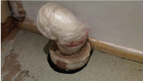
Gaps had appeared in the rubber matting, exposing the concrete lining of the tank to seawater
