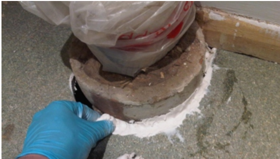
AB Original was kneaded by hand and then pushed into the crack, filling the gap
