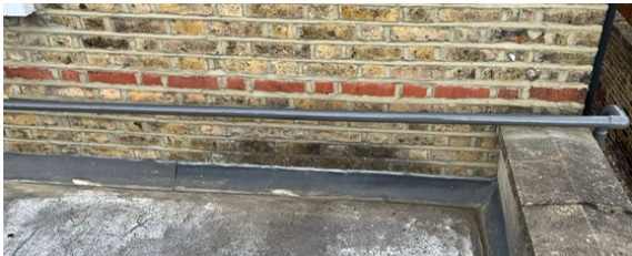
The pipe was painted in Liquid Metal to reinforce and strengthen the brittle metalwork
