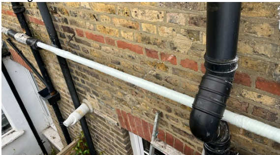
SylWrap Bandage was applied over the Liquid Metal coating, forming an impact resistant shell
