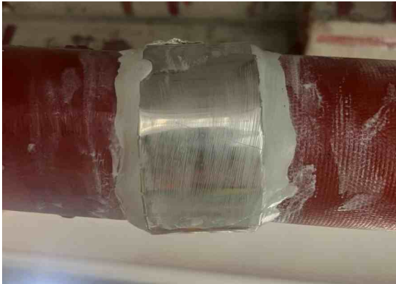
AB Original was forced between repair clamps and the uneven pipe surface, sealing any gaps
