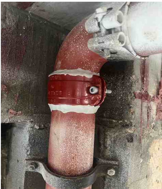
120kg of AB Original was used to seal 300 joints in the rainwater stack before it was blocked back off
