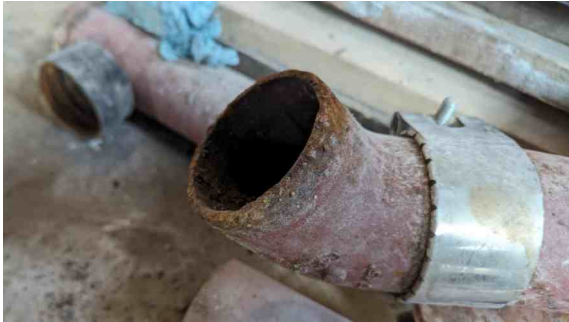
Corrosion had left the pipe ends uneven, making it impossible to create watertight joints using clamps
