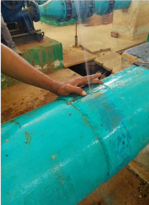
Water had been escaping the 300mm steel pipe for two weeks through a 4mm hole at 6 bar pressure
