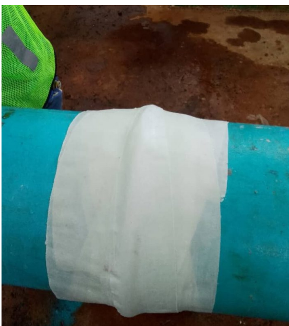
Three 50mm x 11m Wrap & Seals built a repair with enough resistance to withstand 6 bar pressure, followed by reinforcement with SylWrap Bandage
