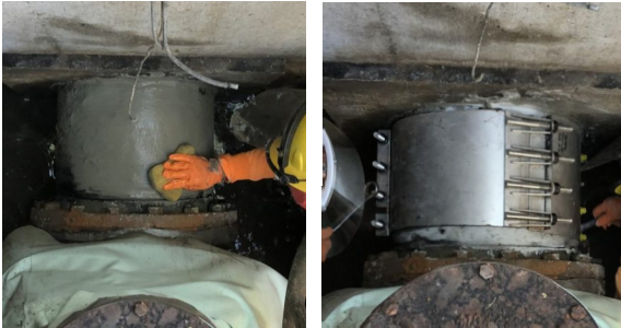
Industrial Metal rebuilt the pipe surface around the hole to make it strong enough to withstand a clamp
