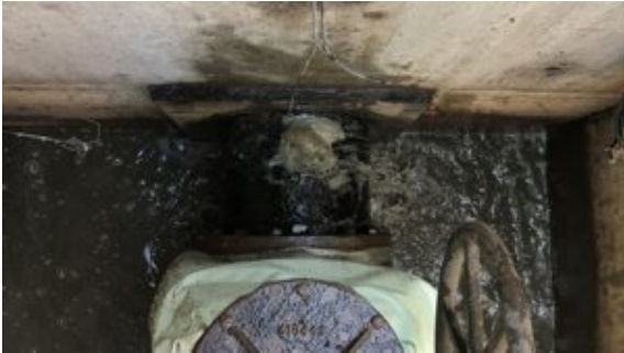
Attempt to clean the pipe by left a hole which water escaped from when the pipe was pressurised
