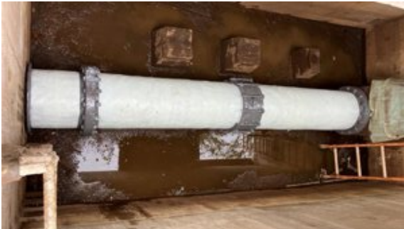
Six layers of SylWrap HD completed the repair by forming a rock-hard, impact resistant shell
