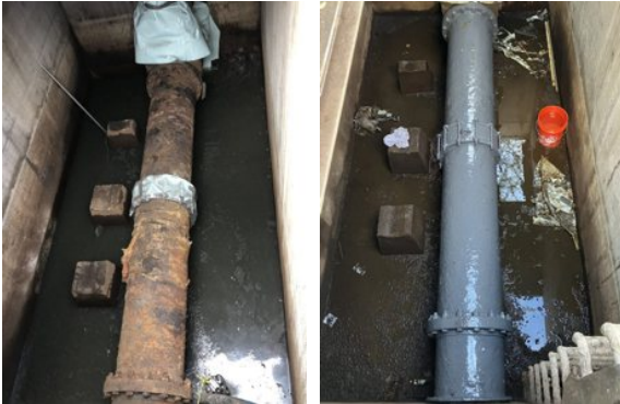
Liquid Metal was painted over the entire main, two flanges at either end and a coupling in the middle to create a metallic external shield against corrosion
