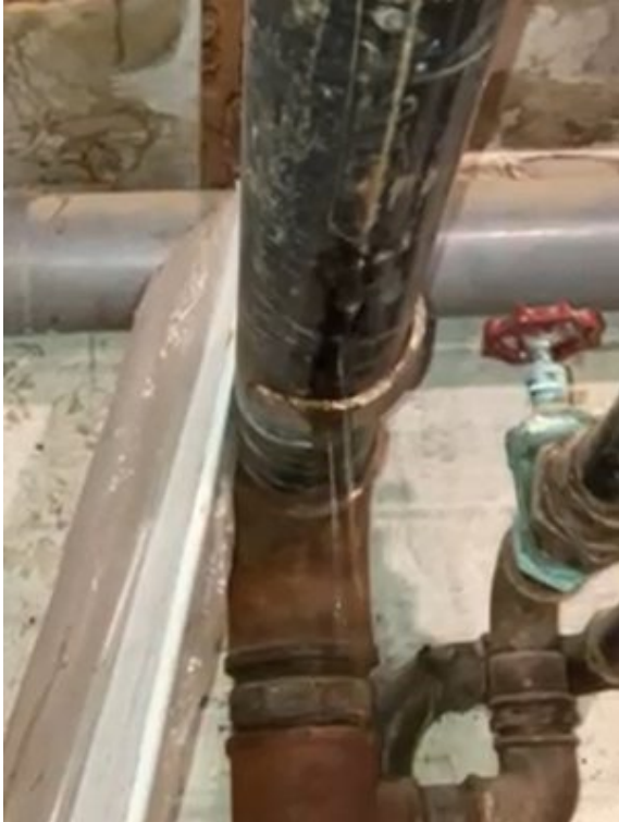
The heating pipe was losing water through a pinhole leak, saturating surrounding loft space
