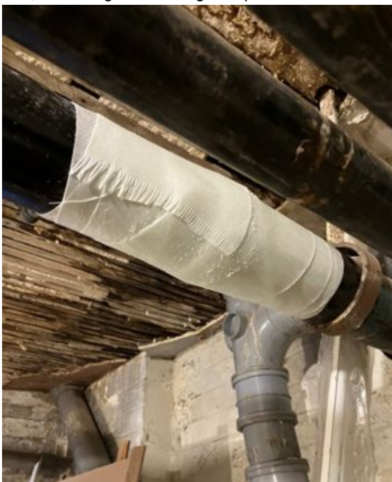
Wrap & Seal sealed the leak before overwrapping with SylWrap HD Bandage for a permanent repair
