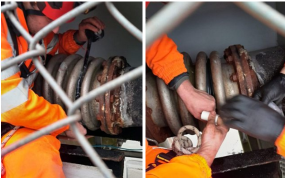
Wrap & Seal was applied between the bellows, covering the split in the expansion joint
