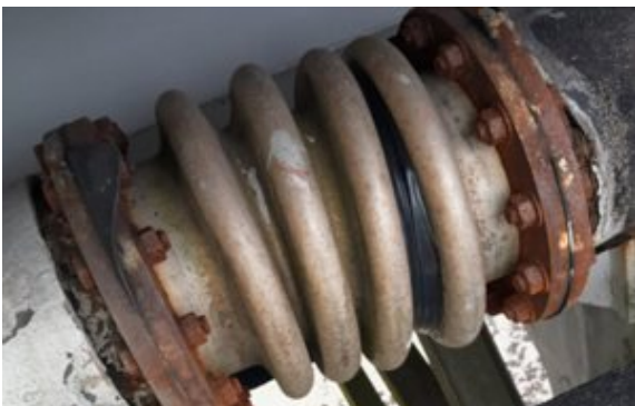
The completed repair left a solid rubber band over the leak, containing pipe content
