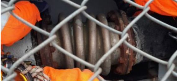
The expansion joint was leaking through a split between the two bent bellows on the right hand side
