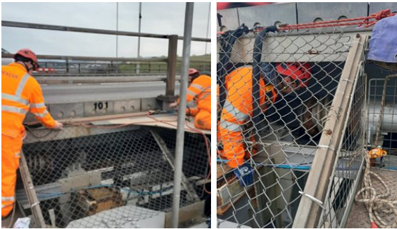
The steel pipe ran beneath the suspension bridge road deck in a severely cramped space, making access for repair difficult
