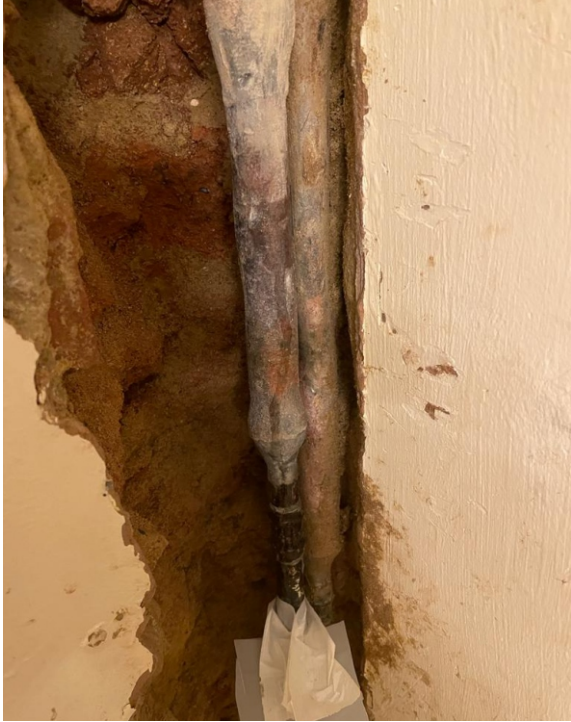
After cutting away the drywall, the homeowner found a leaking vertical 25mm lead water pipe
