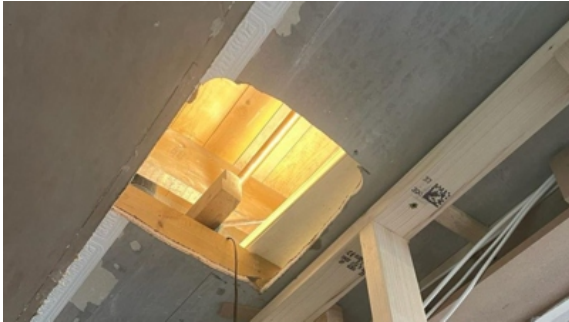
The joint had to be sealed with the pipe in place due to limited access through a small hole in the ceiling
