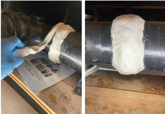
AB Original was formed into three long 'sausages' which were wrapped and smoothed around the joint, leaving it completely covered in a ring of epoxy putty
