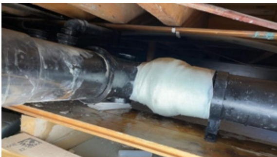
The repair was completed by reinforcing the leaking section with SylWrap HD
